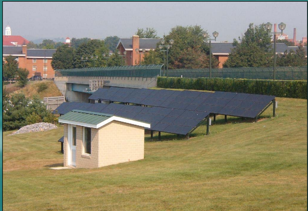
CISAT 10-kW Solar Electric Plant (CSEP)
