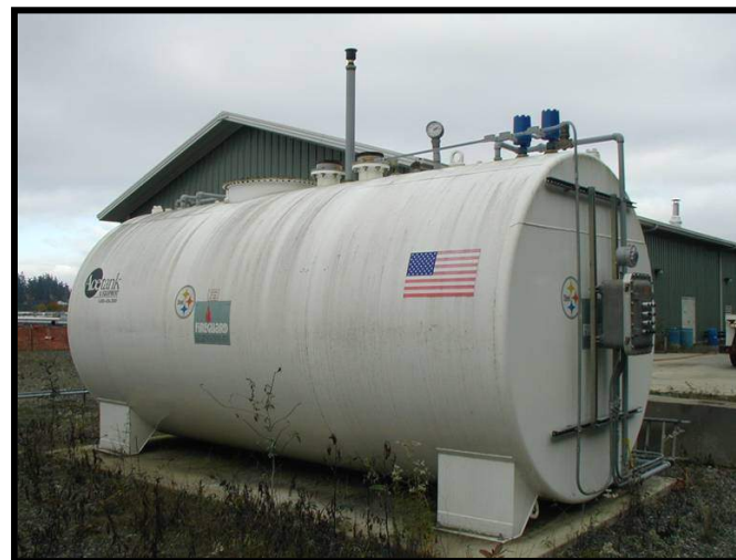
Fuel tank with remote dispensing installed in consumer-hostile industrial location enclosed in fenced perimeter.
